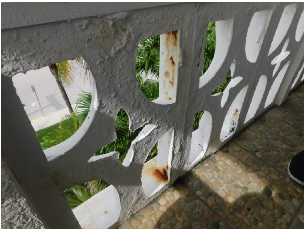
Figure 24. Corrosion staining on the ornamental precast panels.
