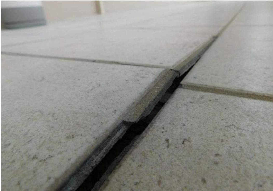
Figure 13. Close-up view of the vertically displaced tile
