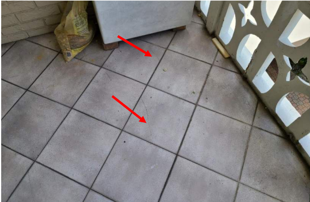
Figure 11. Tile finish cracking
