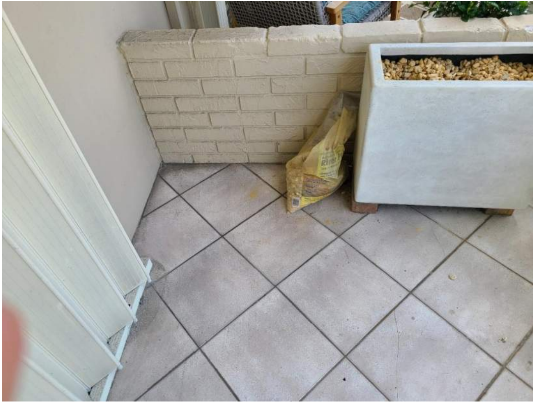
Figure 5. Brick knee wall separating the continuous balcony by unit
