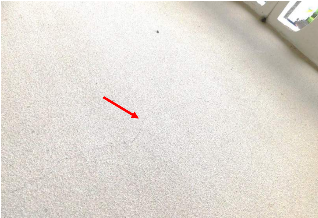
Figure 10. Balcony slab crack
