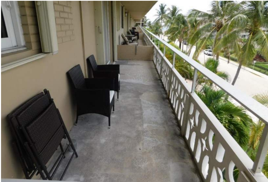
Figure 18. Failed or removed concrete protective coating on deck
