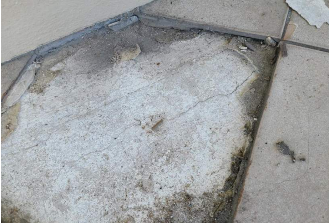
Figure 15. Close-up view of concrete slab cracked and delaminated below tile finish
