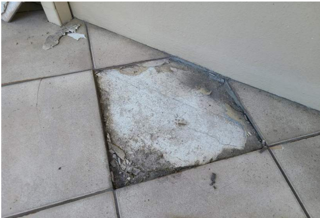
Figure 14. Inspection opening with concrete slab cracking underneath
