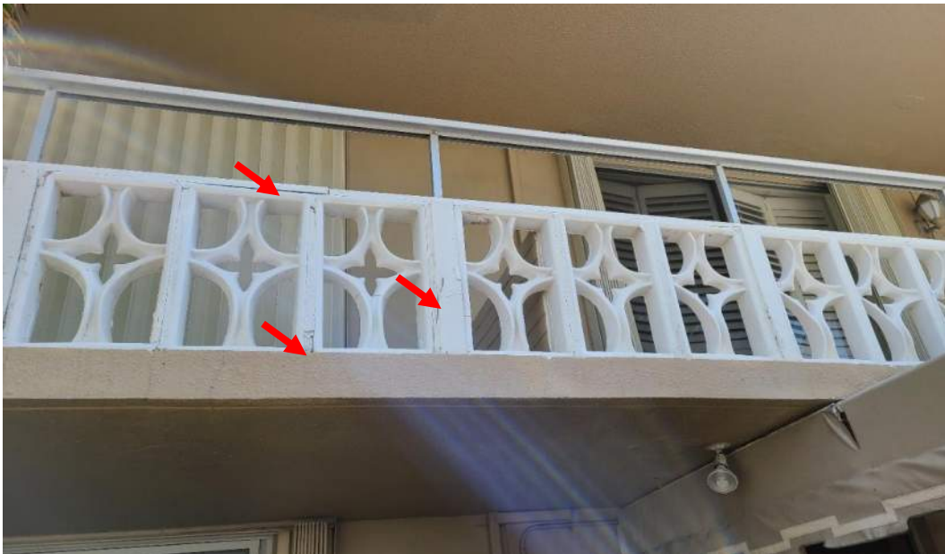
Figure 20. Deterioration of precast ornamental guardrail
