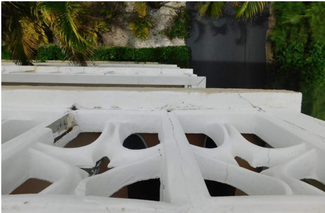
Figure 22. Deterioration of the precast ornamental panels.
