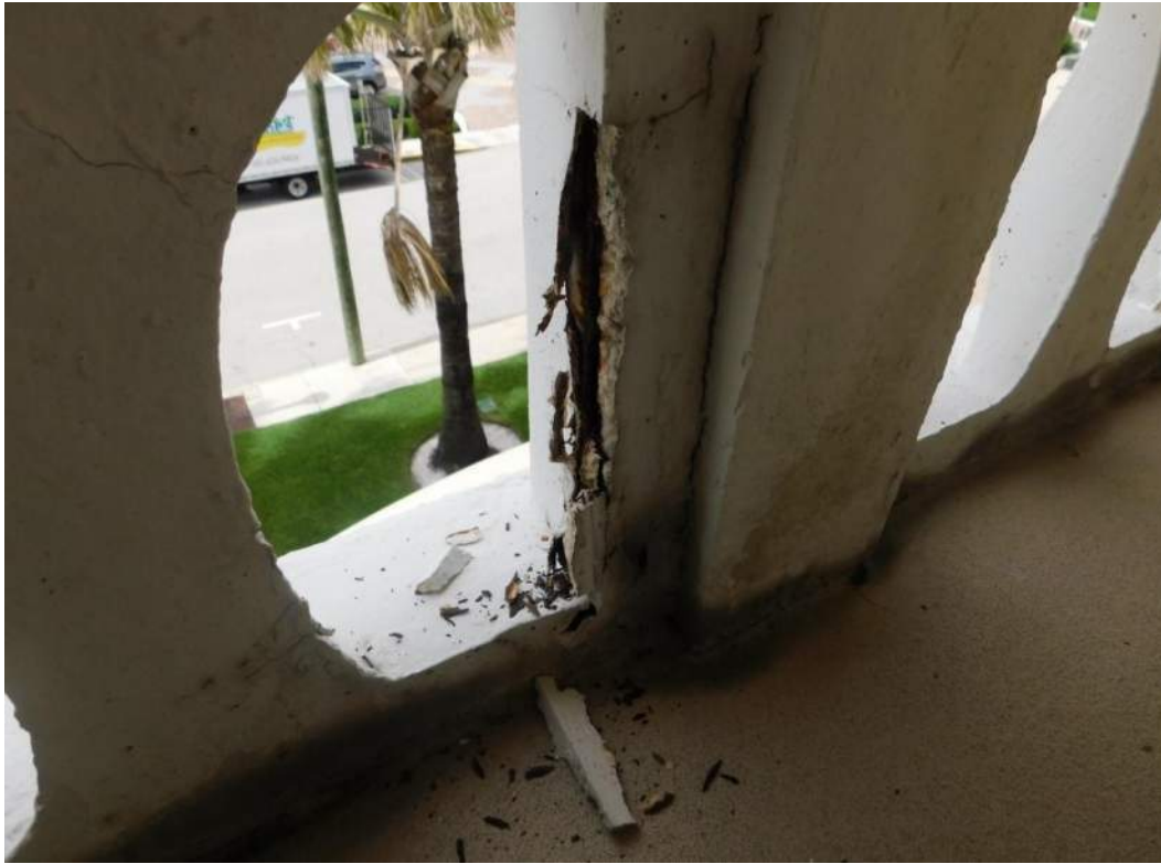
Figure 21. Exposed reinforcement on the precast ornamental panels.
