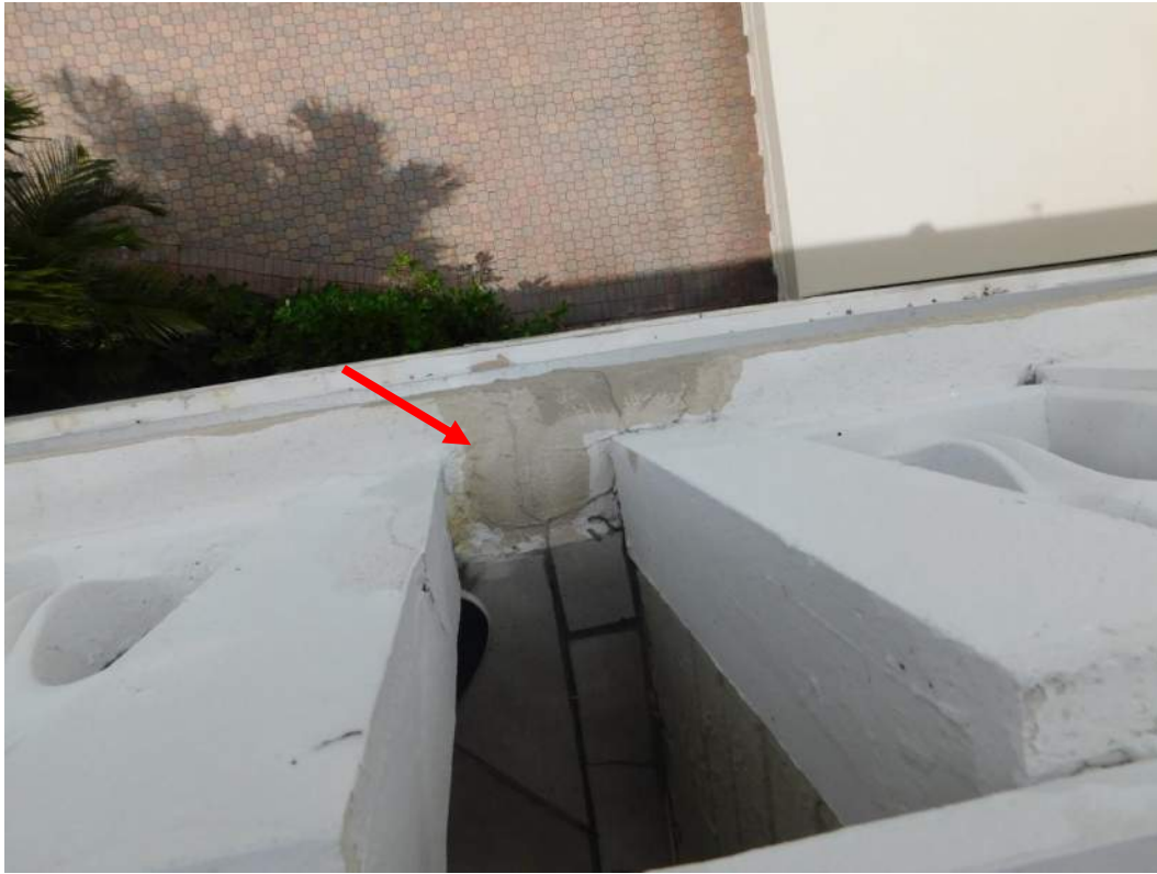
Figure 9. Unsound previous repair
