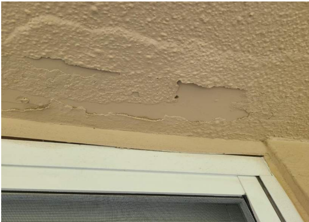
Figure 16. Coating failure on the soffit.
