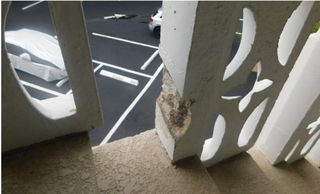
Figure 23. Spalling and exposed reinforcement on the ornamental precast panel
