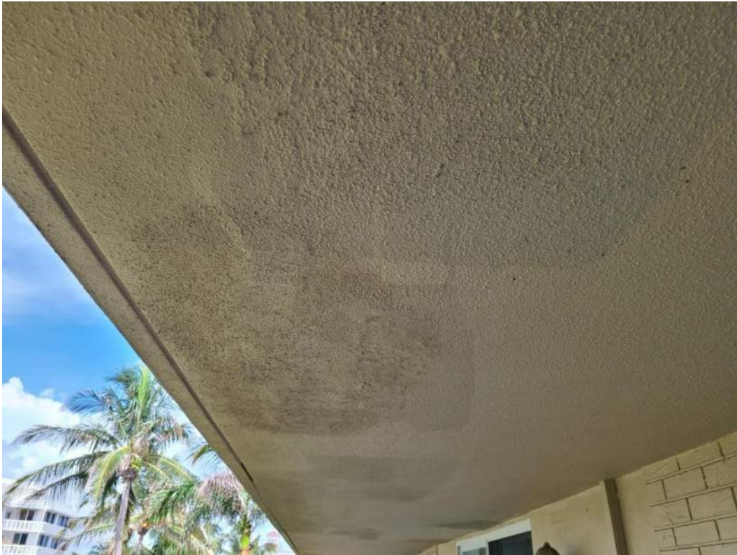
Figure 19. Previous patch repair observed along soffit
