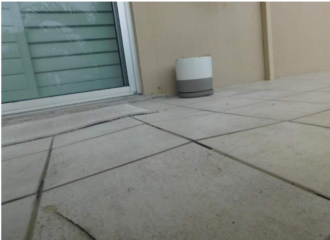
Figure 12. Bowed tile above concrete slab
