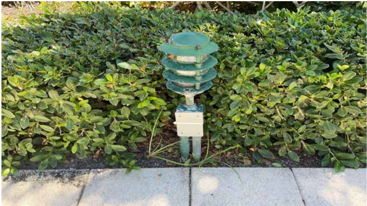
Pool Deck Lighting
