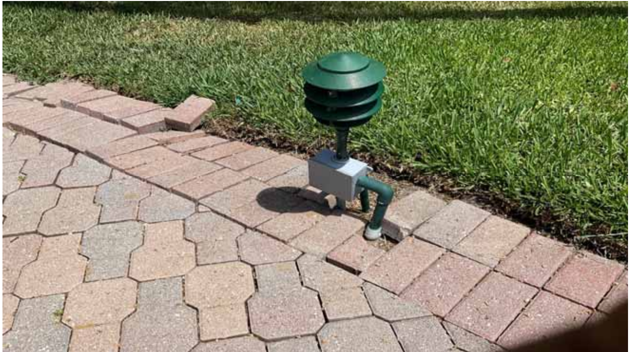
South Bldg Lighting - Parking Lot
