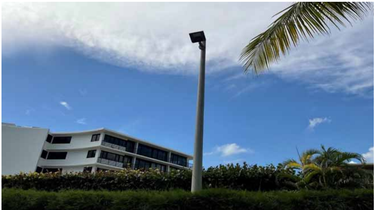
North Bldg Light Pole & Fixture - Parking Lot
