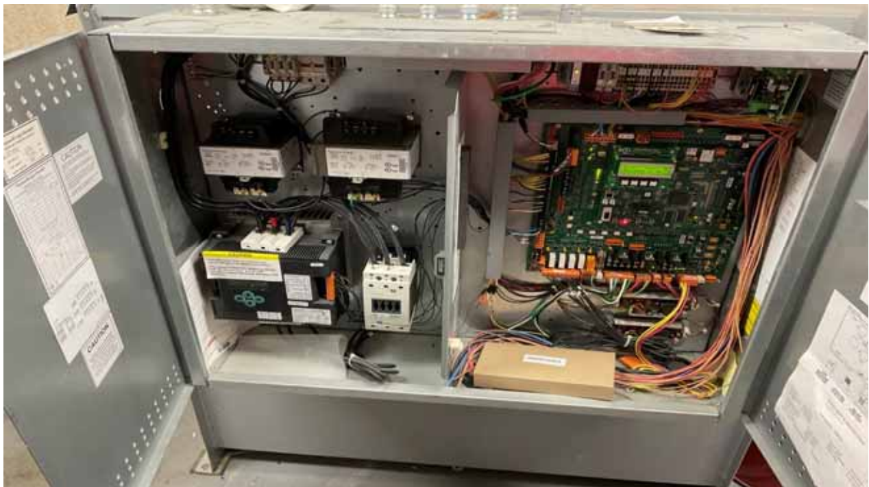
North Bldg Elevator Equipment #1
