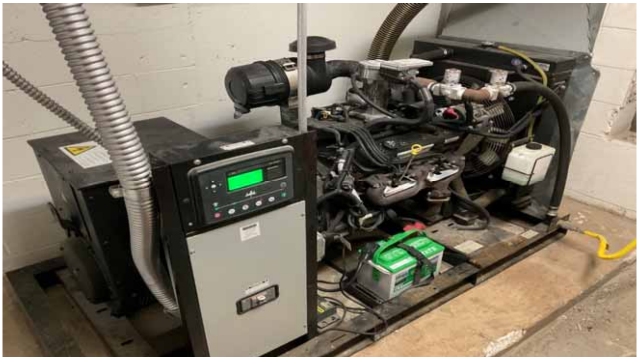
North Bldg Generator
