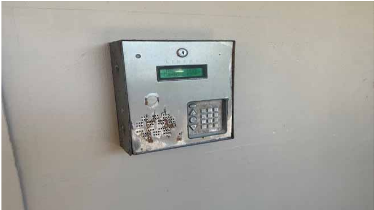
South Bldg Enterphone - Main Lobby Entrance
