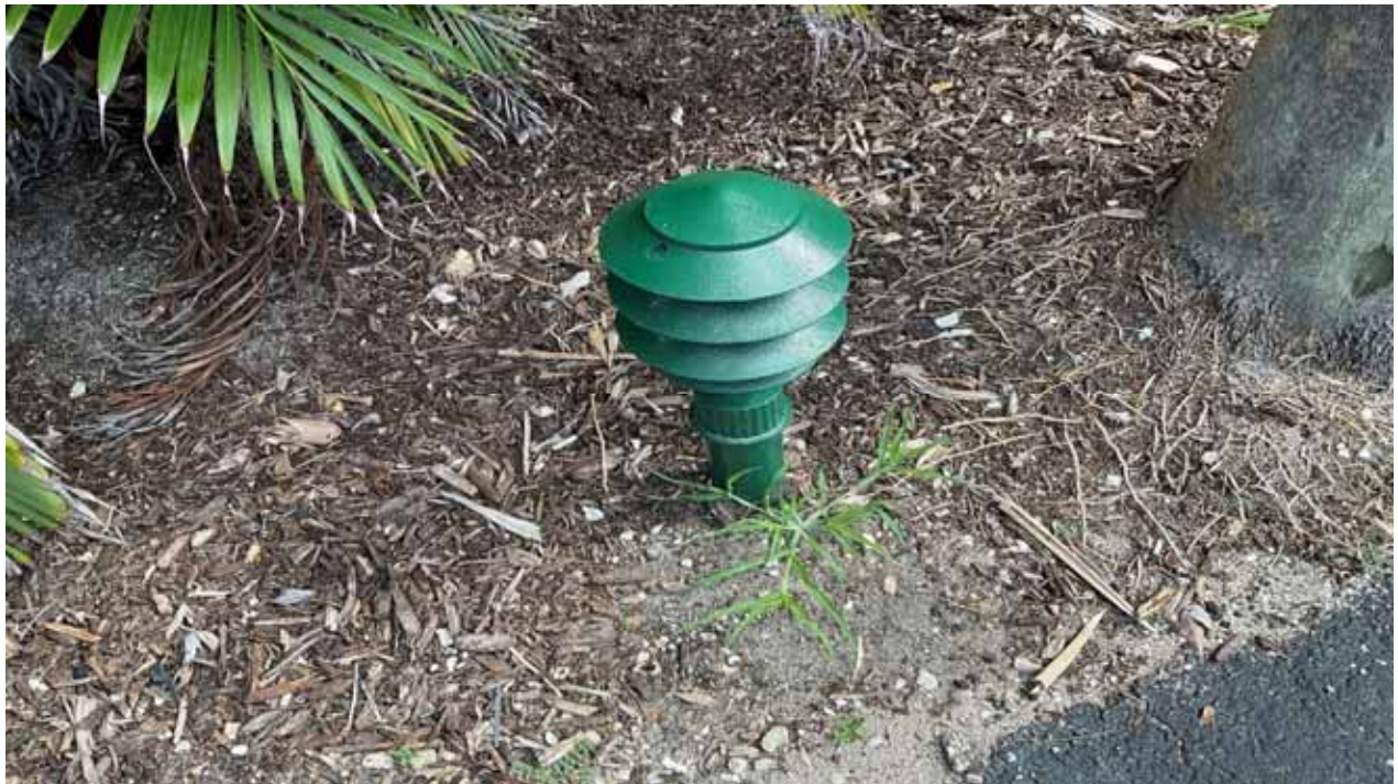
North Bldg Lighting - Parking Lot
