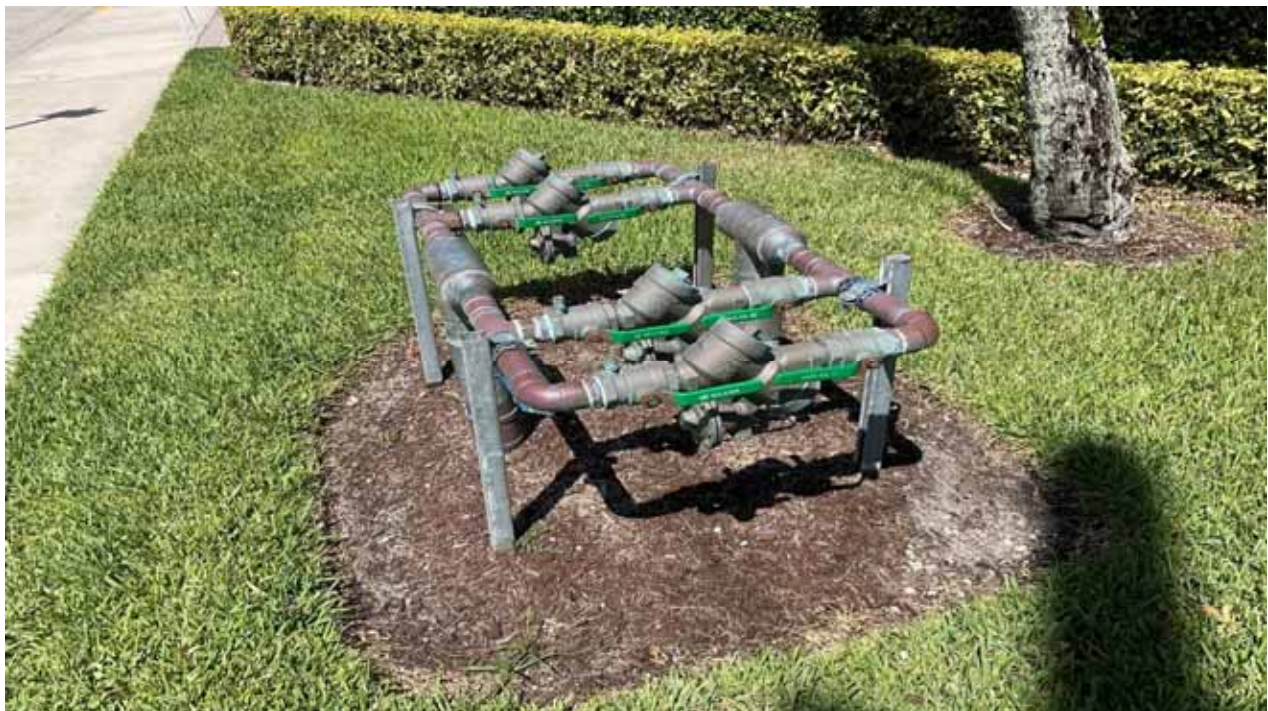
South Bldg Backflow Preventer
