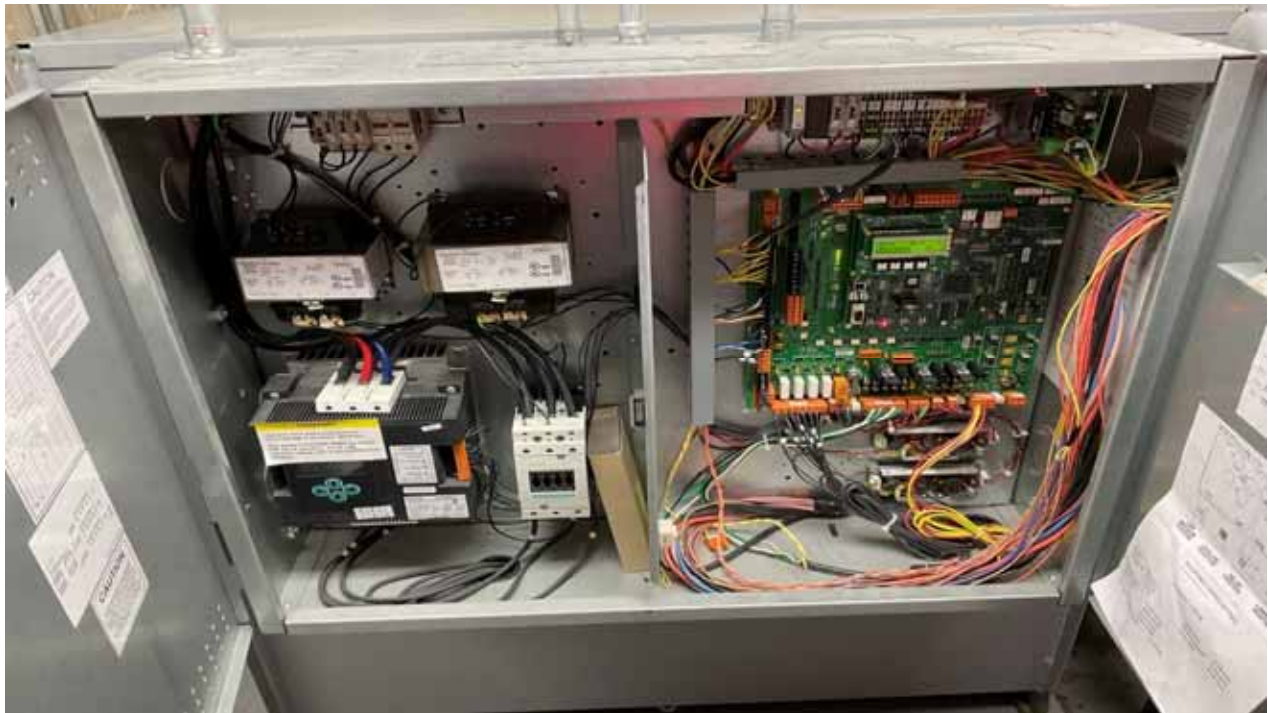
North Bldg Elevator Equipment #2
