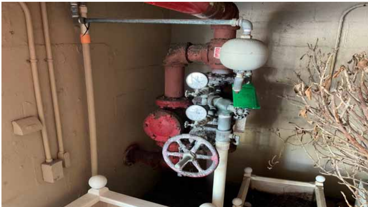
North Bldg Fire Standpipe
