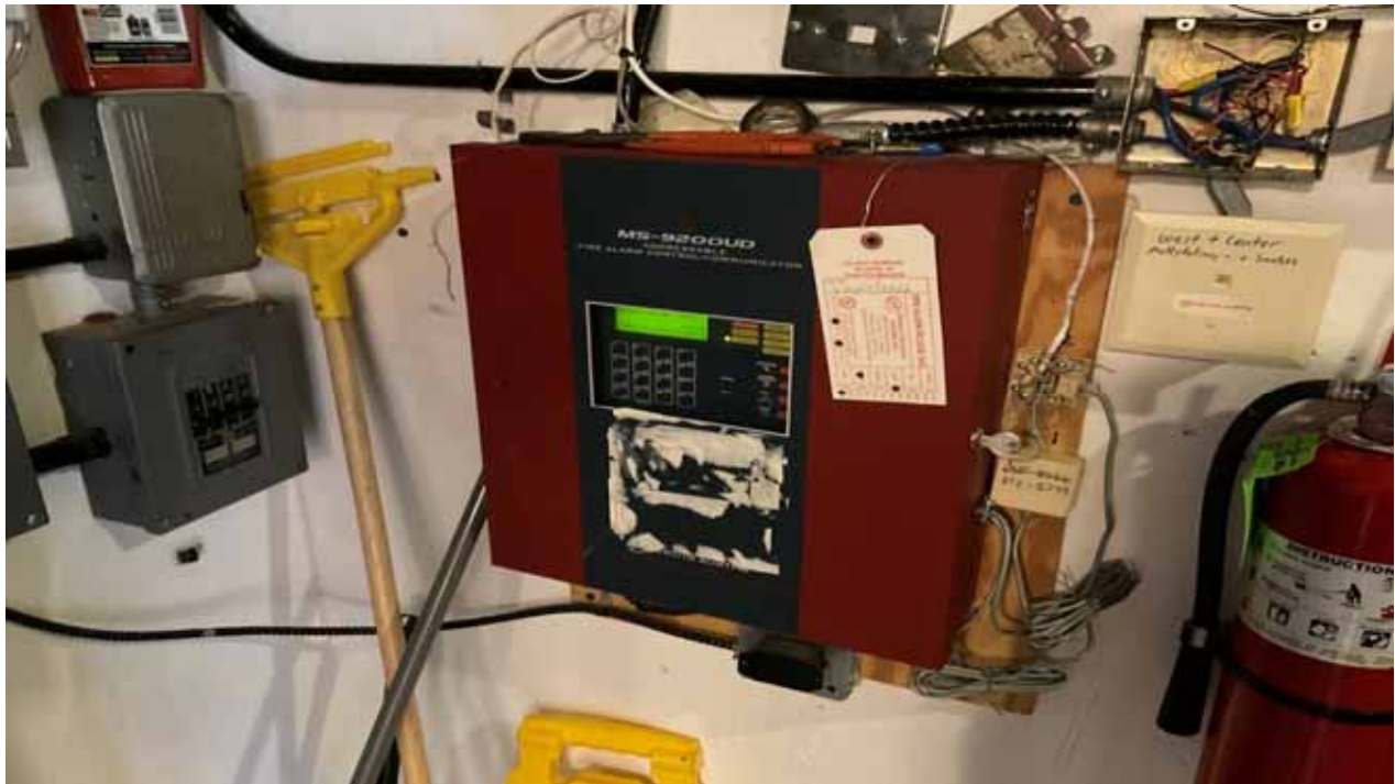
South Bldg Fire Alarm Panel
