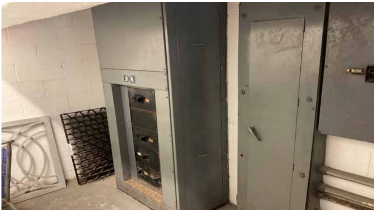
North Bldg Main Electrical Room
