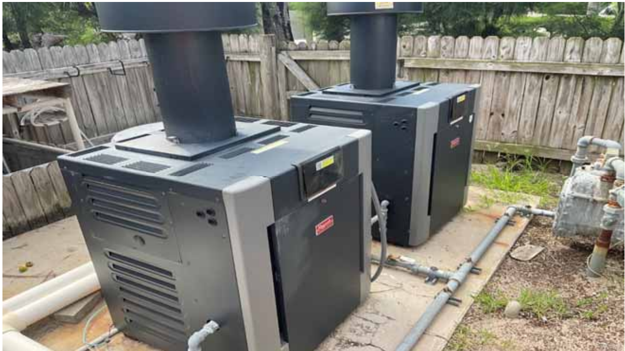
Pool Equipment, Heaters
