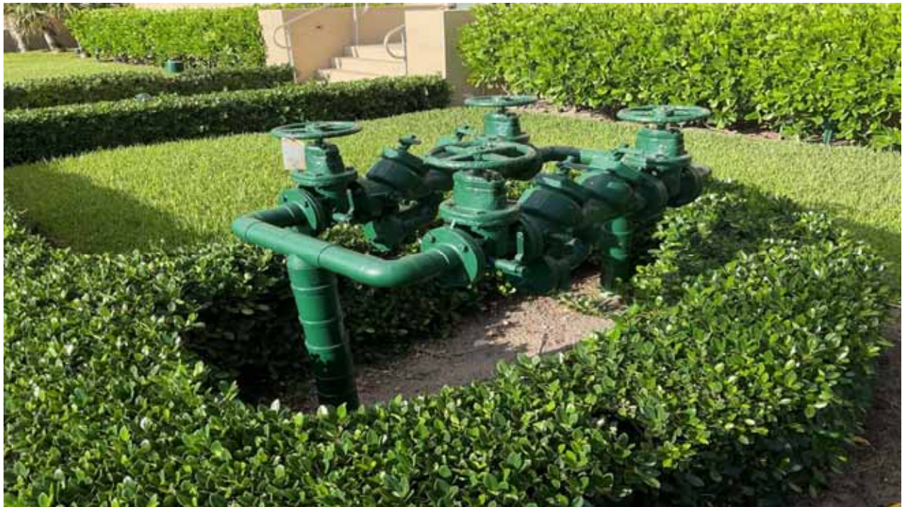
North Bldg Backflow Preventer
