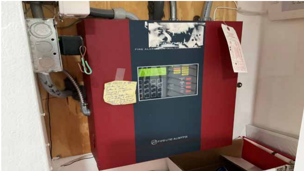
North Bldg Fire Alarm Panel
