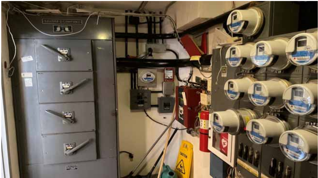
South Bldg Main Electrical Room
