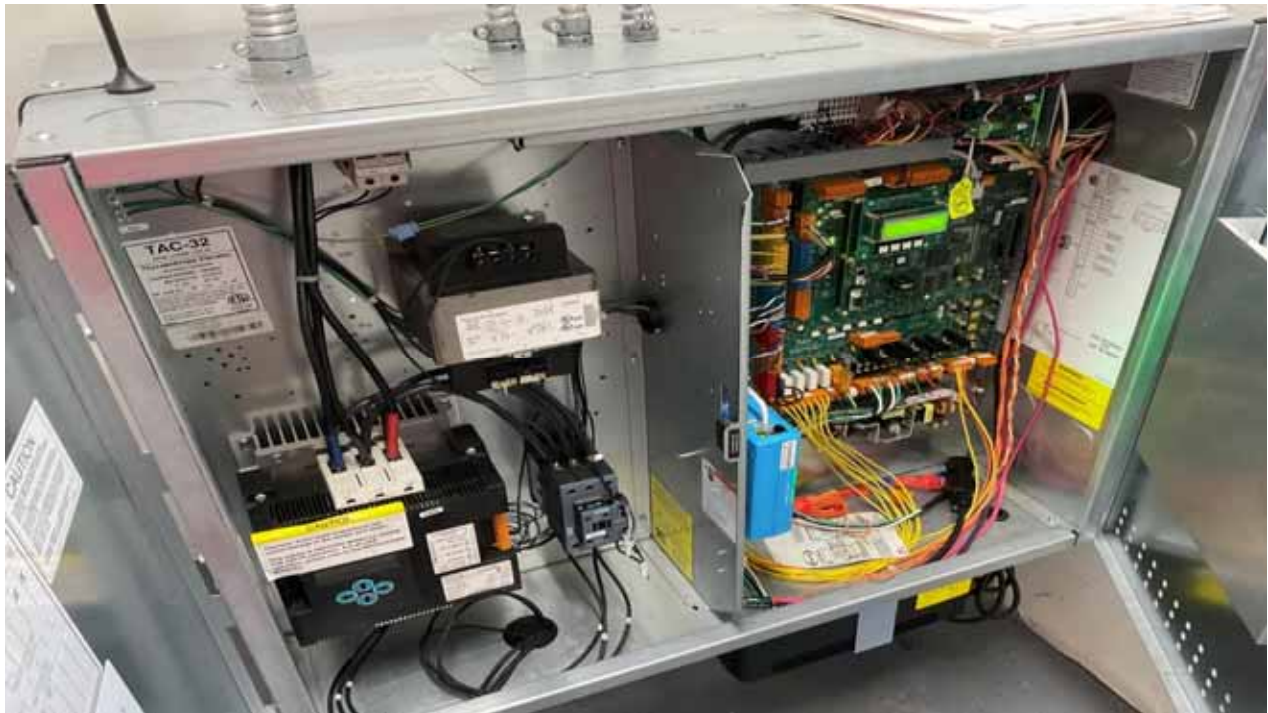
South Bldg Elevator Equipment
