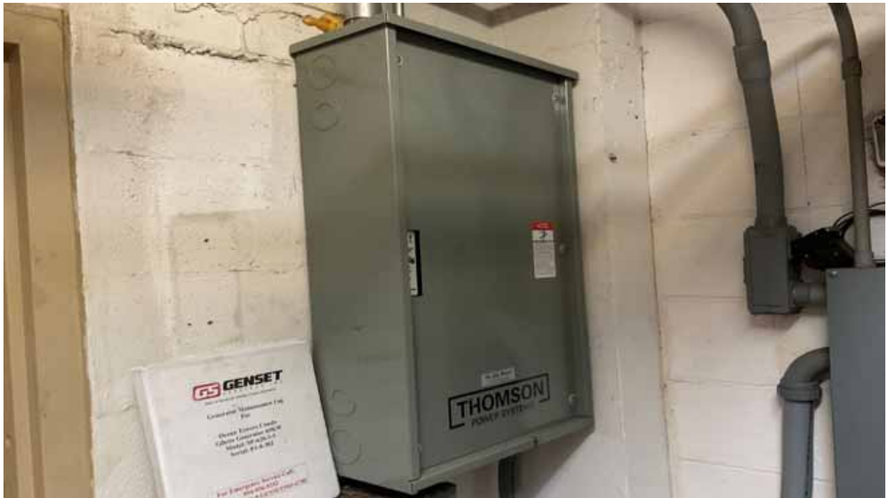
North Bldg Generator Automatic Transfer Switch
