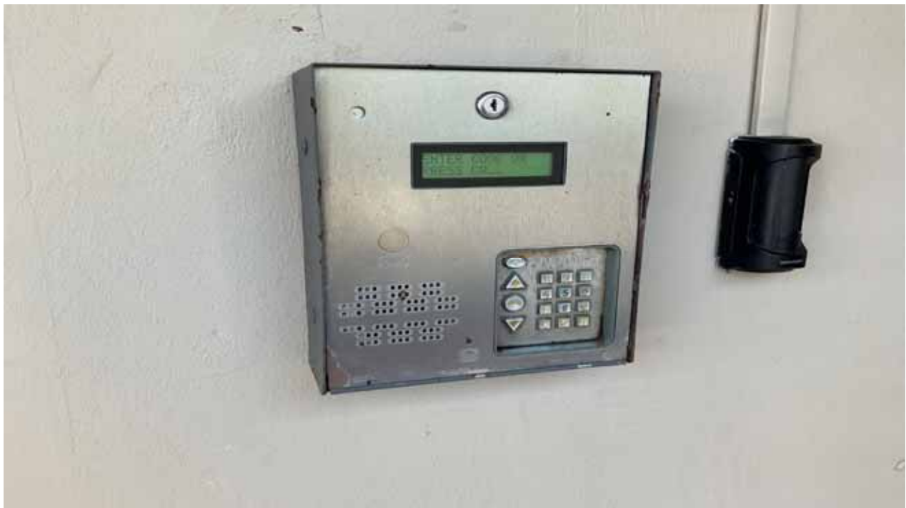
South Bldg Enterphone - North Entrance
